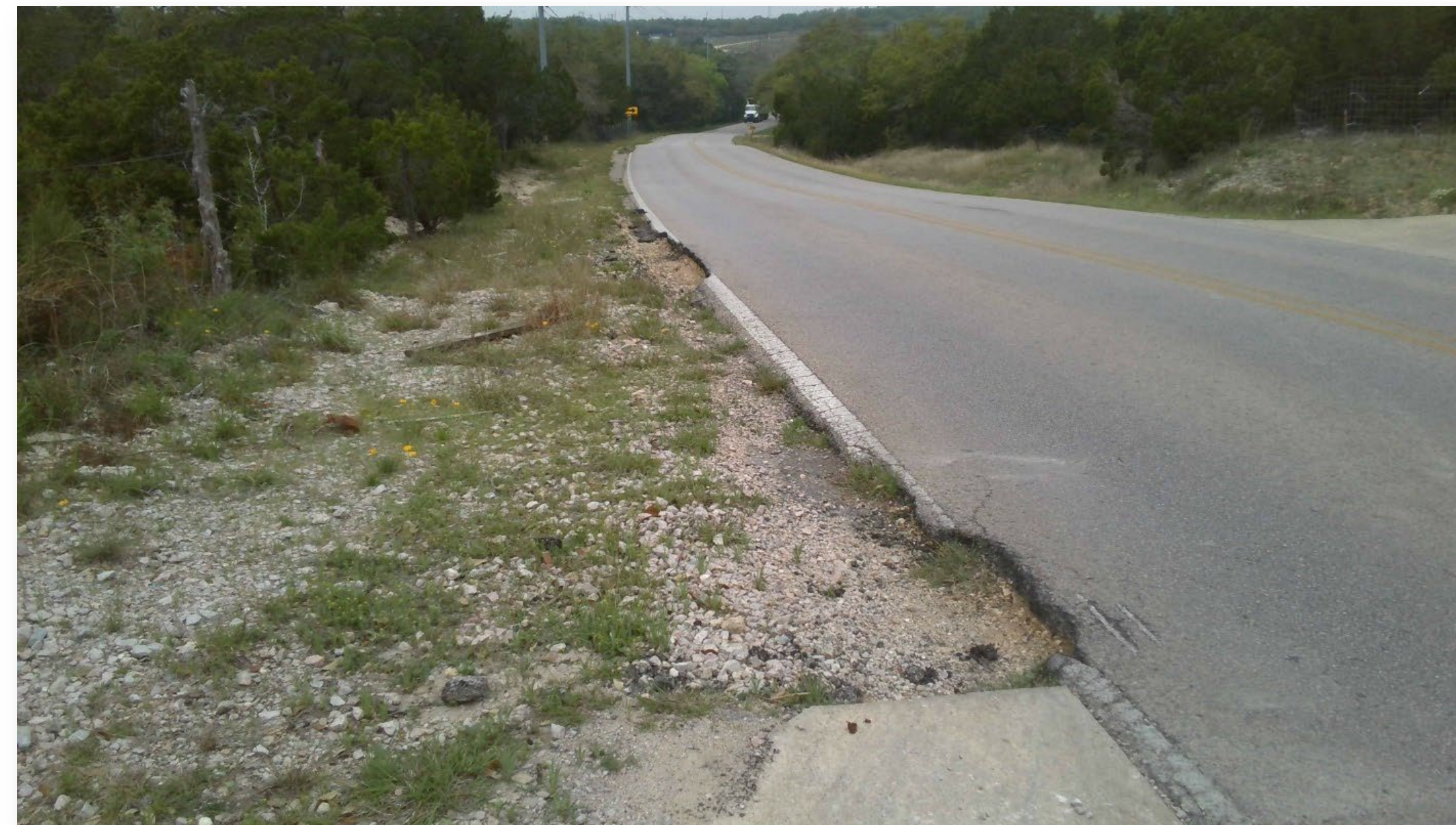
Shoulder & Pavement Marking Deterioration
